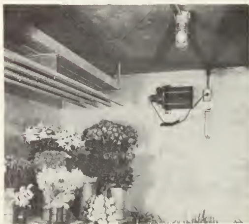
18-13. An activated carbon air filter installed in florist cabinet. Also, note the cooling coils, the hangers and the drains. (W. B. Connor Engineering Corp.)
